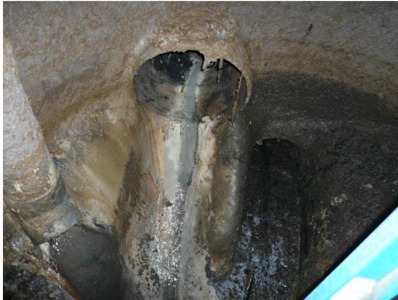
Photograph 4: Base of deep manhole in municipal sewer system coated with moisture tolerant and chemically resistant ARMALINE 1730 epoxy coating. Again, complex shapes require rehabilitation by coating.
