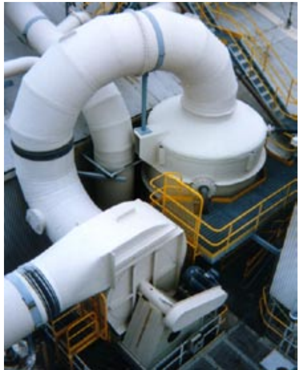
Void tower scrubber at fertiliser works removing fluoride gases with sea water. View shows exit at top of tower and fan in the system.
