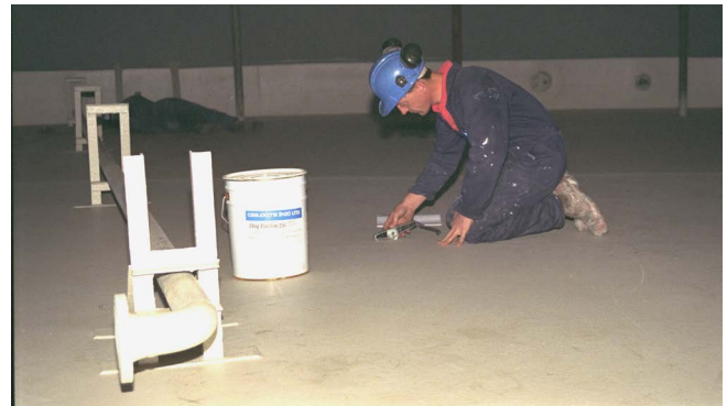
Ceilcote® 200 Series Flakeline applied to base of large storage tank to rehabilitate pitted steel plates and provide long term protection from future corrosion.
