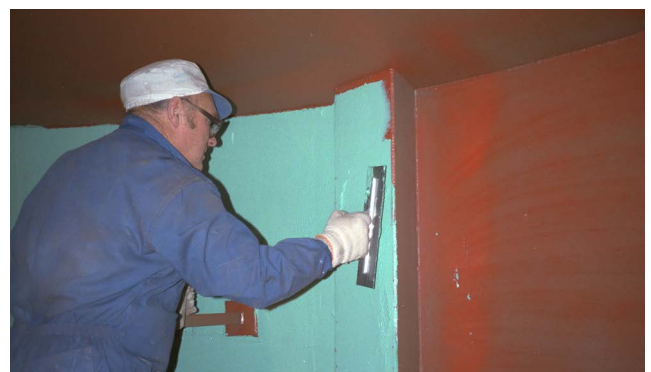
Ceilcote® 100 Series Flakeline trowel applied to inside of chemical steel storage tank used in Pulp & Paper Industry.
