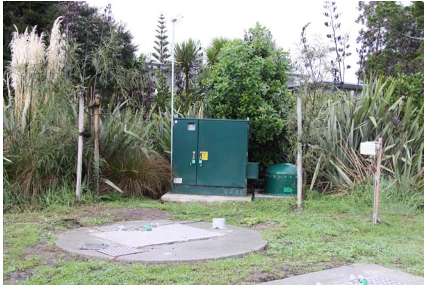
Photo 5: Mangawhai Village Pump Station with 'Green Dome' Passive Carbon Bed Odour Filter
