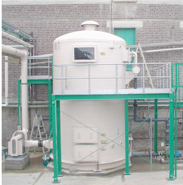
Photo 1: Biological Scrubber At Start-up
