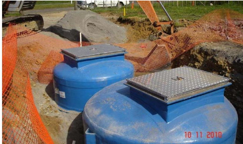
Photograph 18: Eketahuna Fibreglass Pump Station and Fibreglass Valve Chamber
