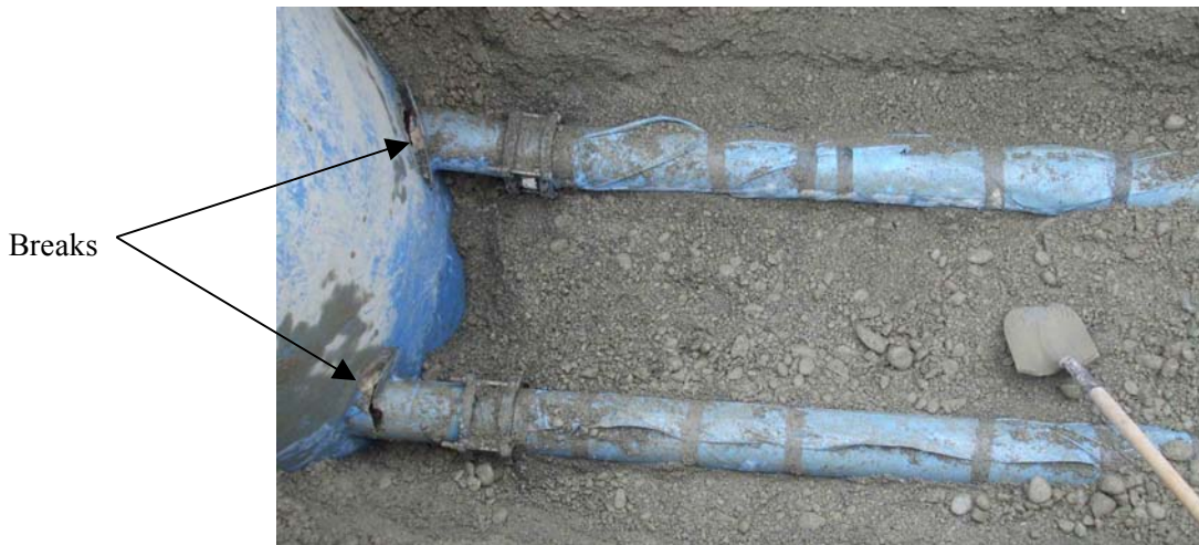
Photograph 16: Wigram Pump Station, Christchurch (PS101): Both 150mm diameter discharge pipes to the valve chamber fractured in the fibreglass pipe spool at the pump station wall.
