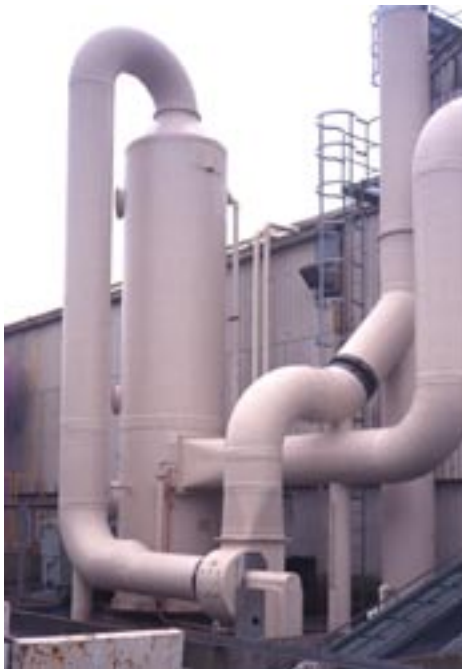
Vertical packed tower removing hydrogen sulphide from air discharge from tannery operation.
