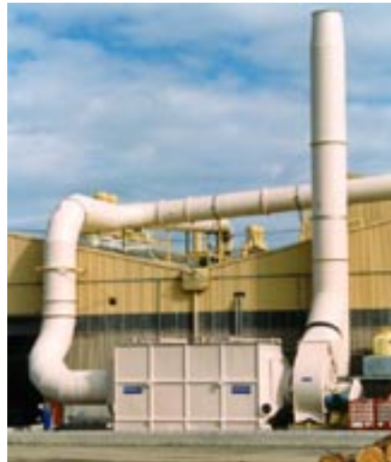
Horizontal crossflow scrubber at particle board plant. This unit has two separate scrubbing beds in series for removing formaldehyde.
