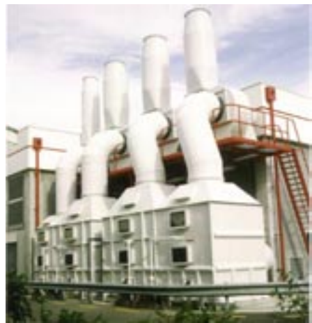
Vertical air washers removing liquid entrainment and fumes from electroplating operation.
