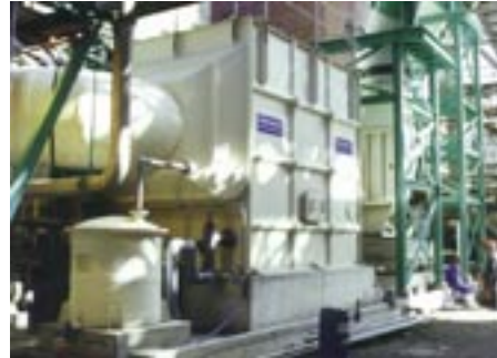
Part of three stage horizontal crossflow scrubber system removing sulphides from gases from black liquor oxidation process at pulp and paper plant.
