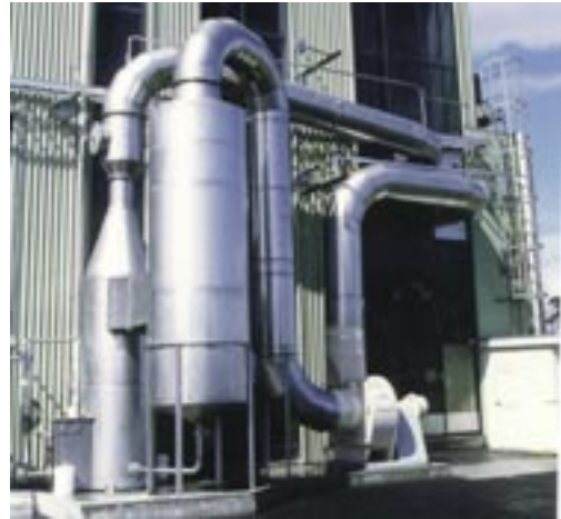
Venturi scrubber and wet cyclone on food product drier
