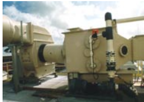
Horizontally mounted multi-throat venturi scrubber removing large particulate from moist exhaust gas stream at a food product drying operation.
