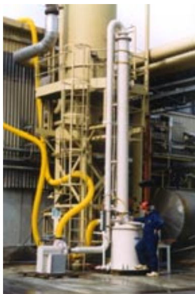
ARMATEC's 300mm diameter vertical counter-current packed tower pilot plant scrubber on trial at an industrial site. Capacity 0.2 m 3 /s.
