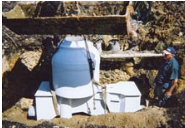
Parshall Flume pre-installed in an all fibreglass manhole being installed in a waste water pipeline during a 9-hour shutdown.
