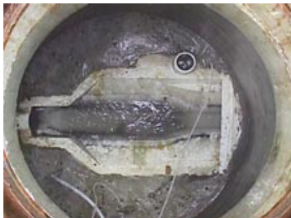
ArmaFlume TZ-150 in operation in a manhole. Measuring and sampling tubes permanently attached so when connecting sampler, personnel do not need to enter the manhole.
