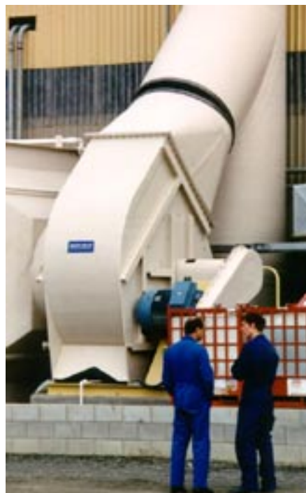
Fibreglass after scrubber at particle board plant
