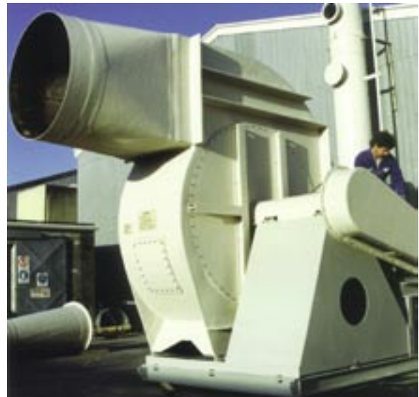
Fan for handling fluoride fumes at fertiliser works.
