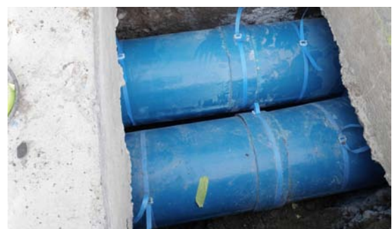
Both 'Carrier Pipes' installed. HDPE pipe is now protected. It has room to move reducing chances of fracture due to ground movement.
