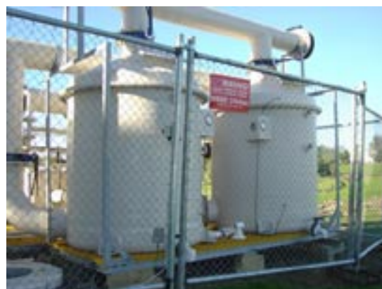
Carbon adsorption beds removing hydrogen sulphide and other odours from landfill gas stream. Fibreglass construction used to handle corrosive airstream.
