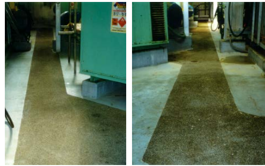
Armaline® Gripcoat on walkway through wet area in Pulp and Paper Plant for personnel safety reasons.
