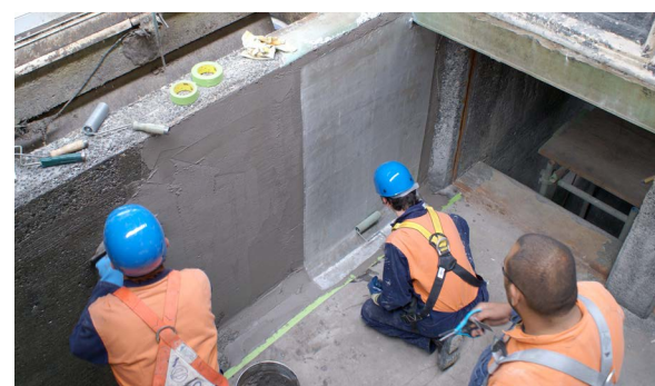
Armaline® 3730 applied to concrete structures and channels in wastewater treatment plant inlet works at Napier milliscreen plant. It has outstanding resistance to hydrogen sulphide gas. The Armaline® 3730 was applied during a tight shutdown period during which water intrusions could not be totally eliminated.
