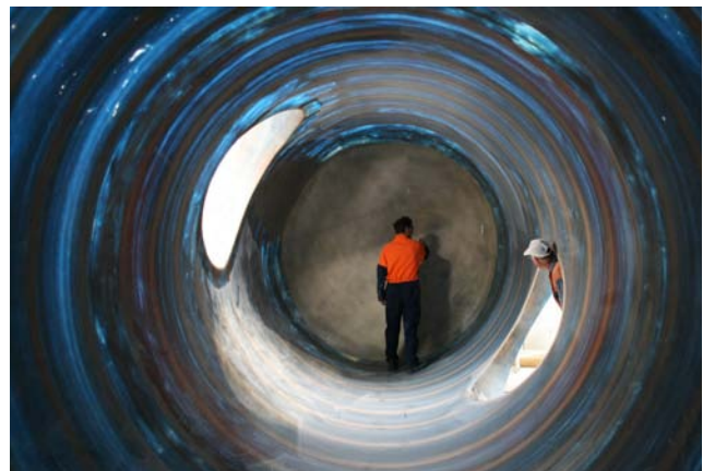
Horizontal surge tank under construction. Pump out chamber is fitted to one end of surge tank.
