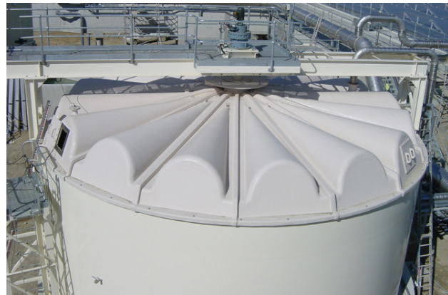
Segmented barrel vault design fibreglass cover for a WWTP thickener at Lower Hutt, NZ.
