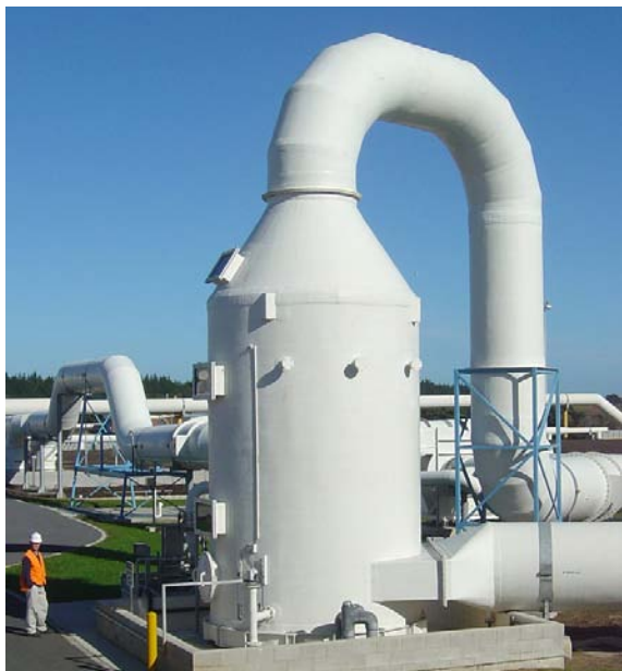
Vertical packed bed scrubber removing ammonia from gas stream, ex biosolids building at wastewater treatment plant.
