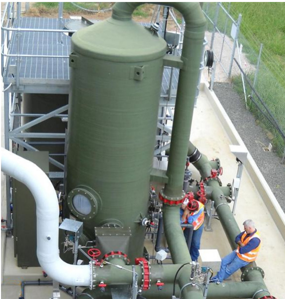
ARMATEC designed biological scrubber removing H 2 S at Sydney WWTP.
