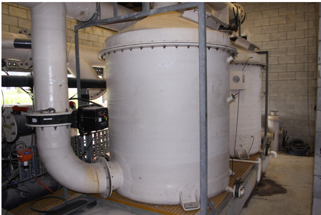
Carbon beds adsorbing H 2 S odours from landfill gas stream.
