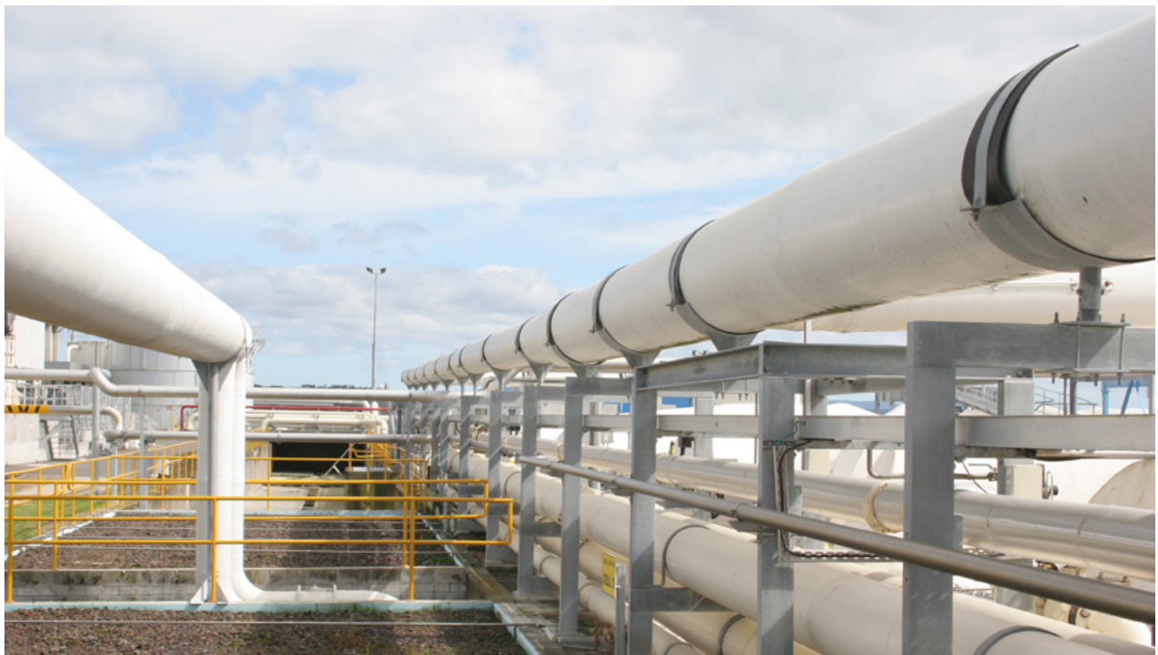
Top: Complete system at food processing plant, treating odours and particulate. Bottom: Fibreglass duct network taking odours to soil bed filters.
