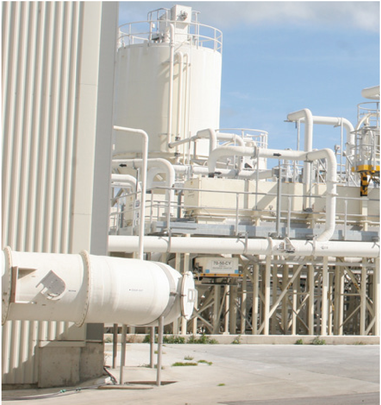
Ventilation system continues from photo at right. Large main duct (front left) connects to main ventilation and scrubbing system. Note manual damper for balancing air flow rate.
