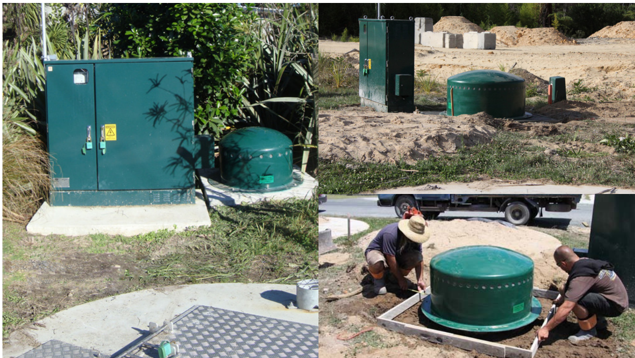
"Green Dome" carbon bed adsorbers for H_2S odours. Passive ventilation - no fans.
