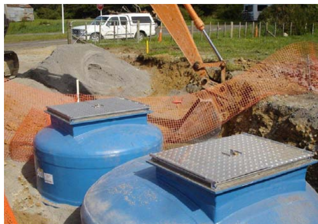
Fibreglass valve chamber (rear) to match fibreglass pump station.
