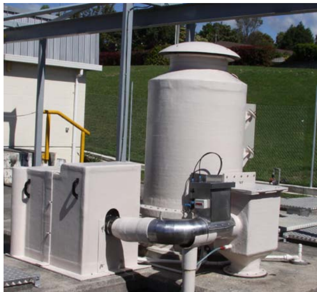
Carbon bed adsorber on municipal pump station. System includes pre-filter, heater for humidity control, fan in acoustic enclosure, and carbon bed adsorber.
