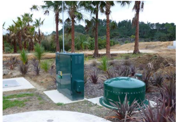
Green Dome™ Odour Filter on pump station vent. No fan. No power. No moving parts.
