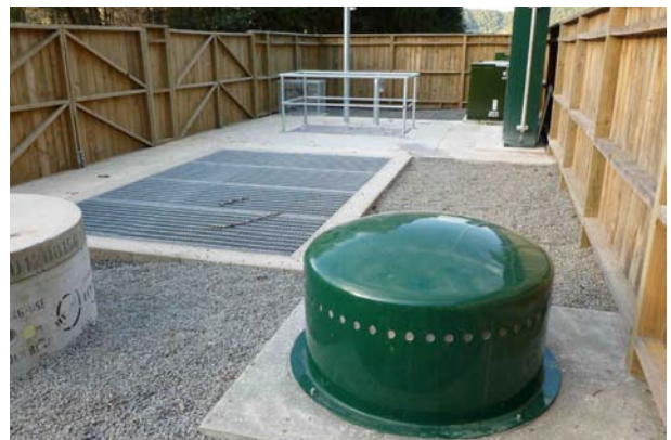
Green Dome™ Odour Filter on pump station.
