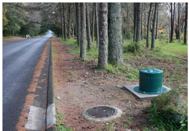
Green Dome™ Odour Filter installed on vent from air release valve
