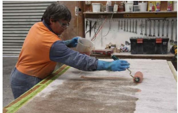
Contact moulding: applying resin to the glass mat reinforcing (CSM - chopped strand mat).
