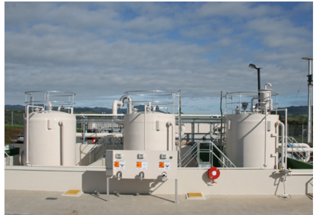
Chemical tanks for wastewater treatment plant, storing sodium hydroxide, alum and sulphuric acid
