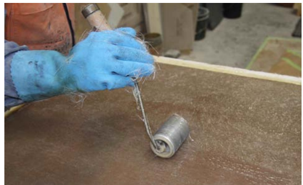
Consolidating the laminate with a ribbed roller to remove air bubbles and achieve physical properties.
