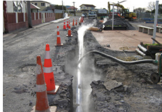
High temperature fibreglass pipe installed through geothermal area. Contract and photo by Hydrus Engineering Consultants.
