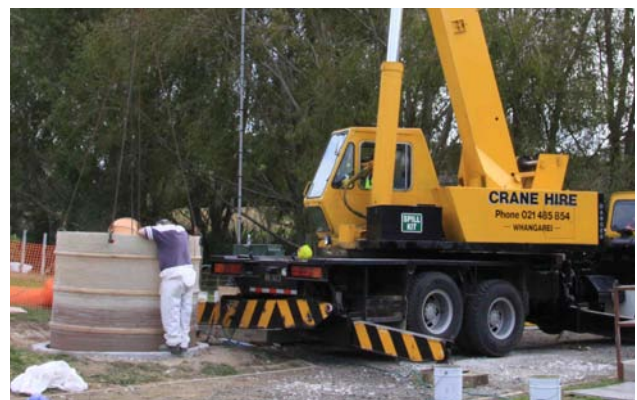
Lowering FRP Liner into place. The top of the manhole has been removed, and the underside is coated.
