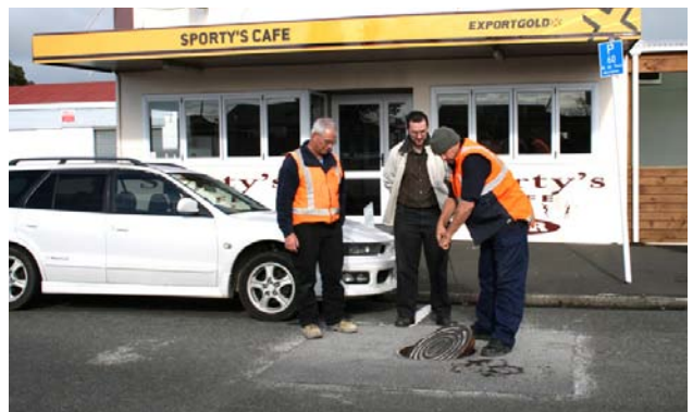
Just four days and a few square metres of excavation was needed to install a FRP Liner in this manhole. If the manhole had been replaced, extensive disruption including road and bar closure would have occurred.
