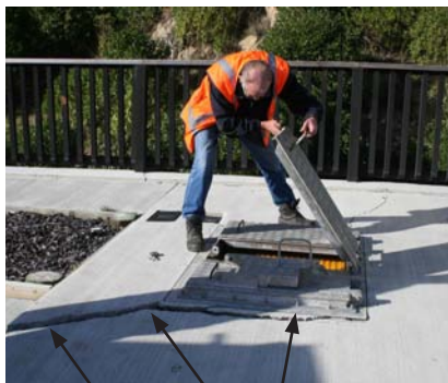
Cracks in concrete.
